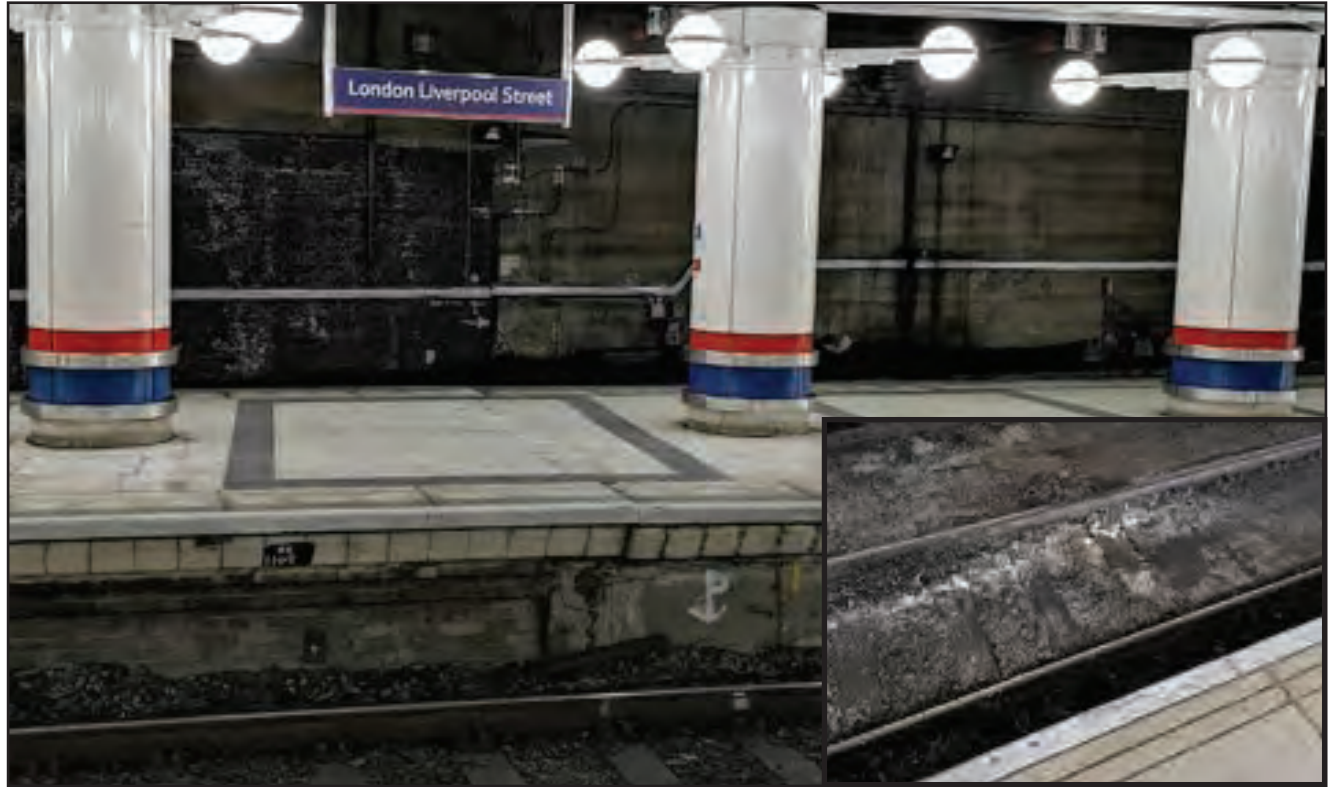
Platform area at Liverpool Street Station (main image). Sewage on tracks (inset image).
